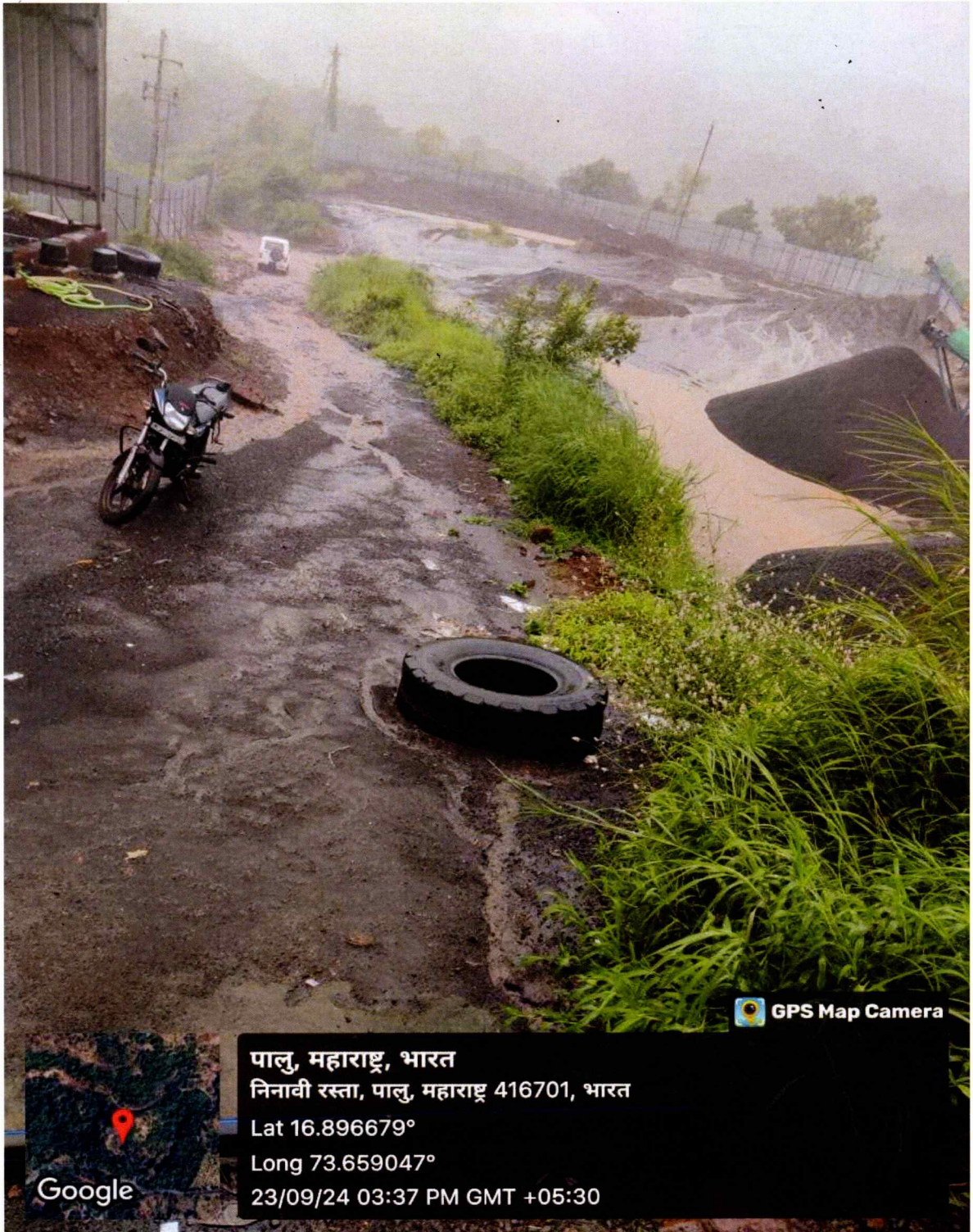
Photographs showing of existing metallic road are ruptured due to rain
